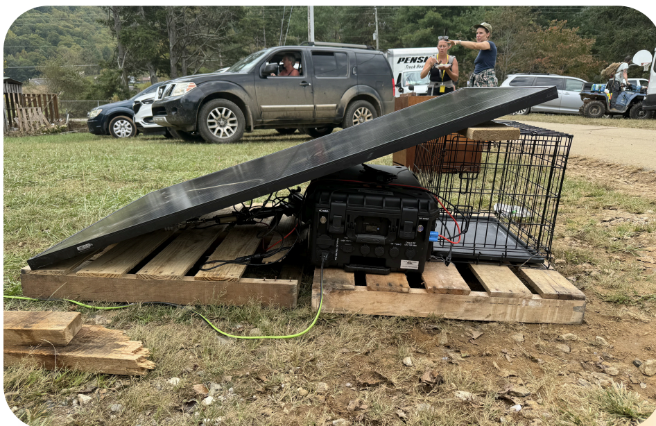
Footprint Project sets up solar panels at Big Ivy Community Center after Hurricane Helene.
